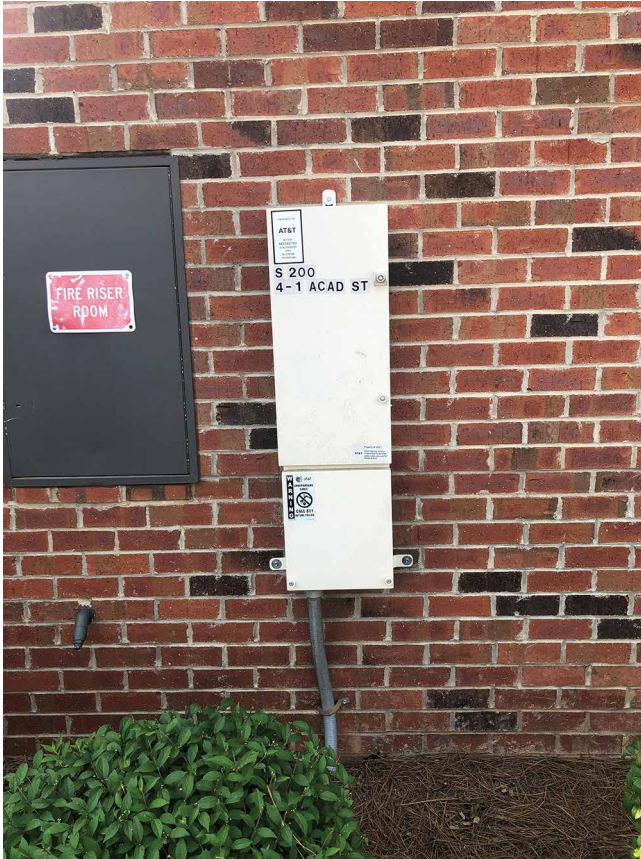
Figure 10. Splitters in Outdoor Cabinets
