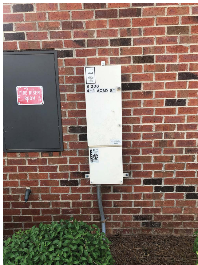
Figure 11. Splitters in Outdoor Cabinets
